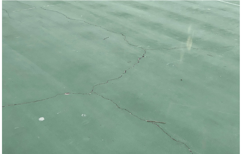
Figure 2. Drying shrinkage cracks in a slab-on-grade originating from the mid-sides and meeting at the centre.
