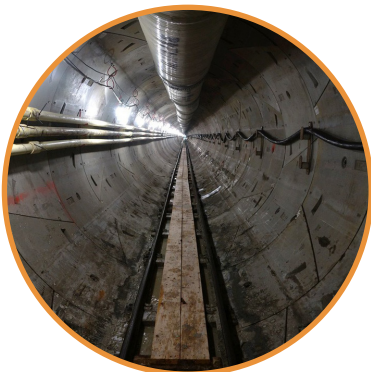
BarChip reinforced segmental lining.
