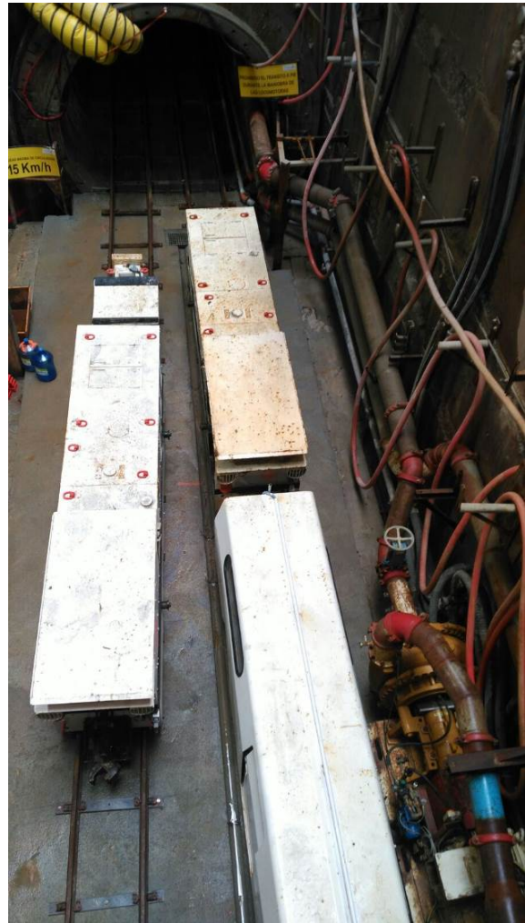
Figure 19. Double track, extraction pump and pipes located in the bottom level of the shaft
