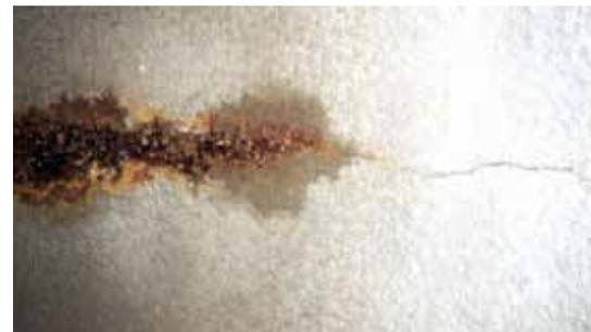
Image 1: Cracking in concrete leads to ingress of corrosive materials, resulting in rapid corrosion of steel reinforcement.
