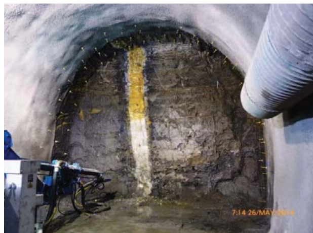
FIG 3 – An 800 mm wide dyke in tunnel face.
